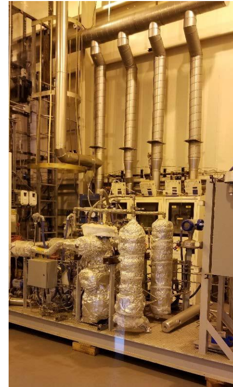
Photograph of the skid installed at SRI (December 2018)
